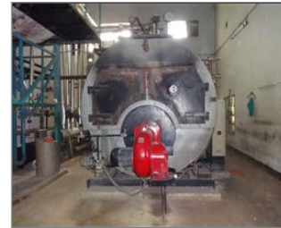
Photo of the inside of the main production hall Boiler room.JPG
