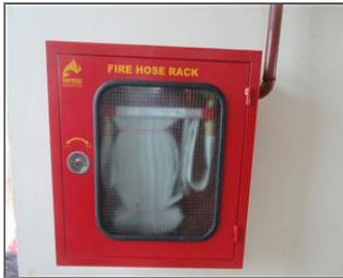
Photo of the inside of the main production hall Fire hose reel.JPG
