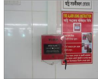
Photo of the inside of the main production hall Fire alarm switch.JPG
