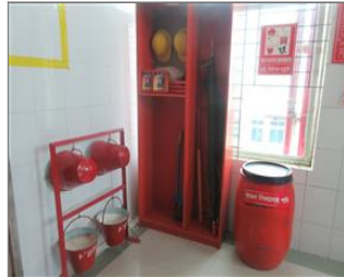
Photo of the inside of the main production hall Fire fighting equipment.JPG
