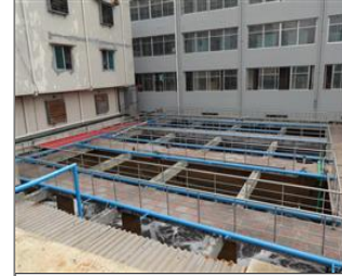
Photo of the inside of the main production hall ETP area.JPG
