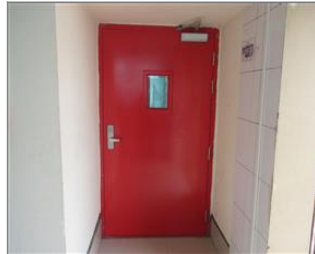
Photo of the inside of the main production hall Fire door.JPG
