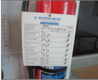
Photo of the inside of the main production hall Fire extinguisher checking card.JPG
