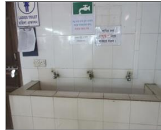
Photo of the inside of the main production hall Drinking water facility.JPG
