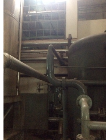
Boiler room unprotected opening
