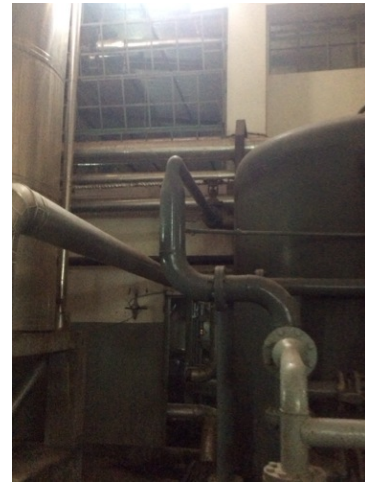
Boiler room unprotected opening
